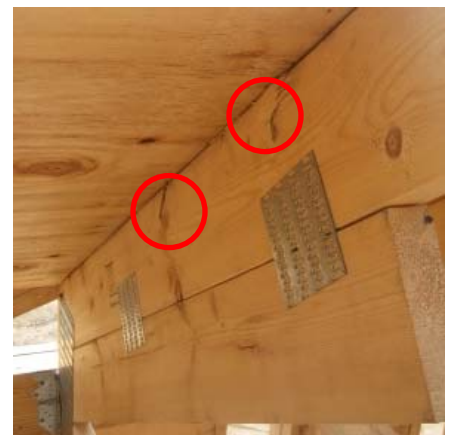
Picture 11: Highlighted missed nails.
